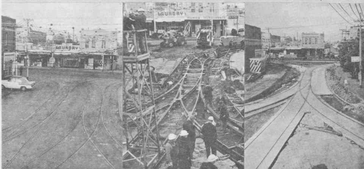
A "before, during and after" composite of the reconstruction of the run-in at Malvern Depot. The centre photograph was taken during the first weekend of major work when the southern turnout was installed. For the following week, cars used only these curves and during the next weekend the northern curves were laid. (Photos. Bob Prentice)
