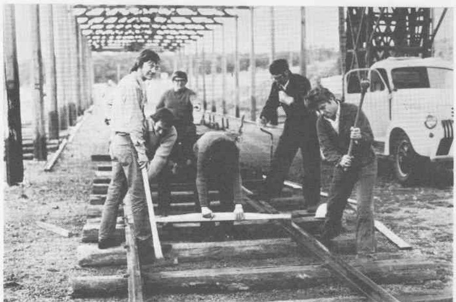
7: At ground level the track team are laying 2 road under the supervision of George Wilcock, the museum caretaker and former VR ganger.
